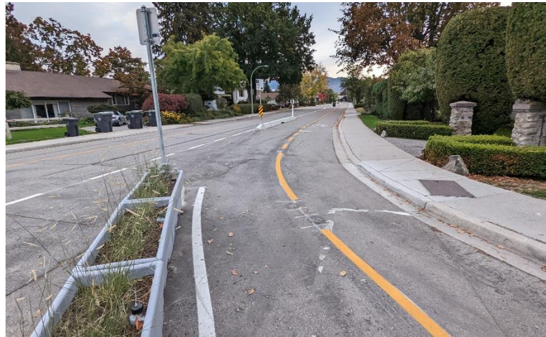
Example of a quick-build two-way protected bike lane in Kelowna, BC using line painting, planter boxes, and jersey barriers.
